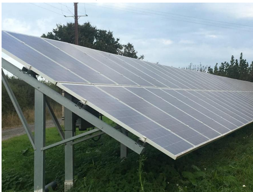
Plate 2-1: Illustrative Array of Solar PV Modules
